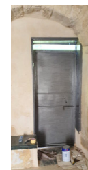
step 2: The window was removed and the door was installed in building no 2
