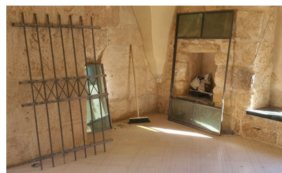
step 1: Dismantling the window protection and frame to open a door in building no 2
