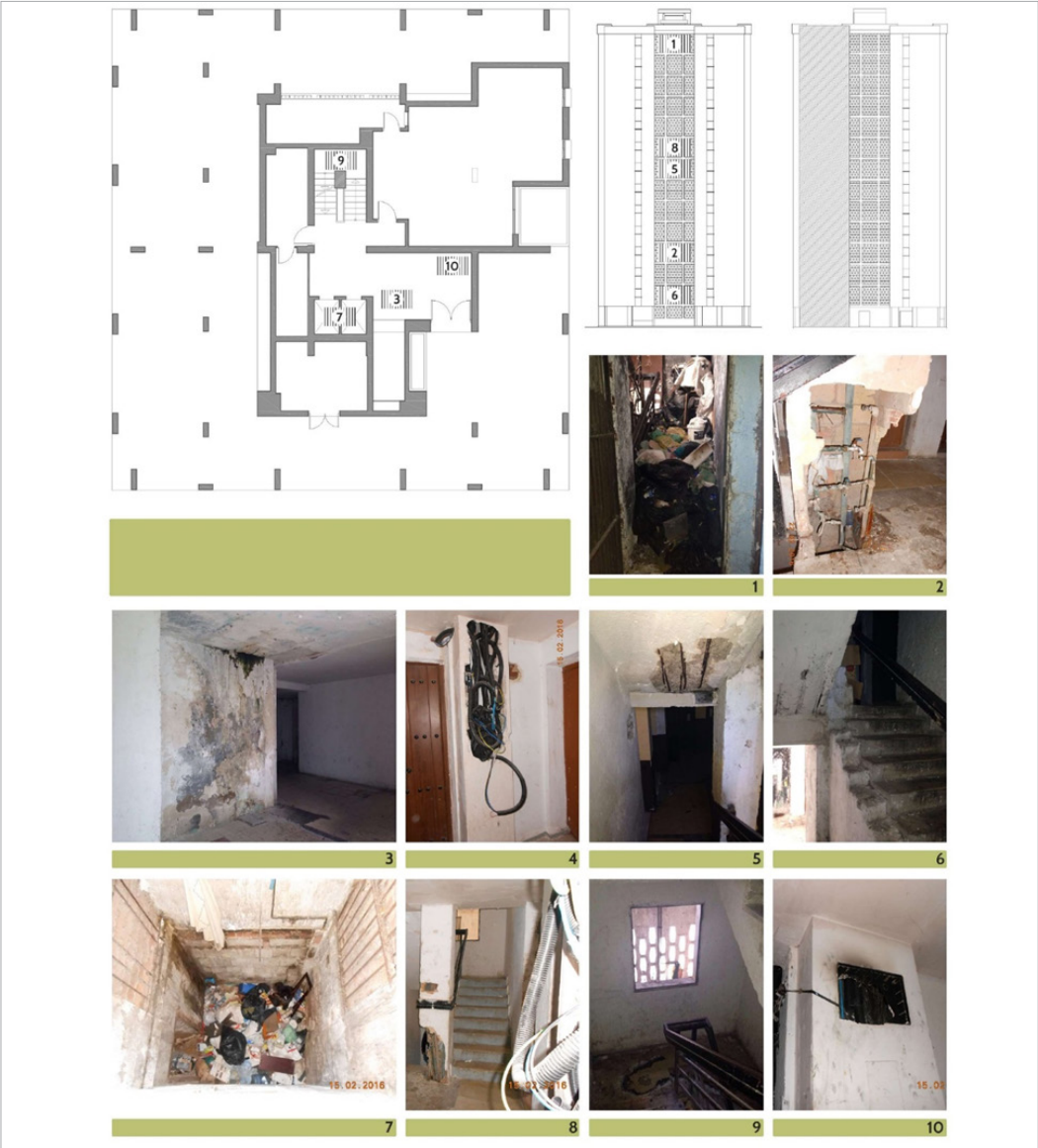
Fig. 5 Location of the main construction defects in the building
